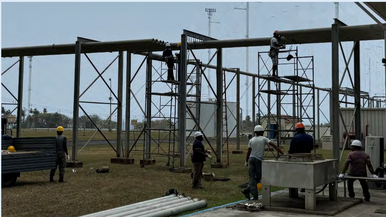
Work crew in Sao Tome dismantling transmitter cabling from USAGM shortwave radio towers and antenna systems (seen in background).
